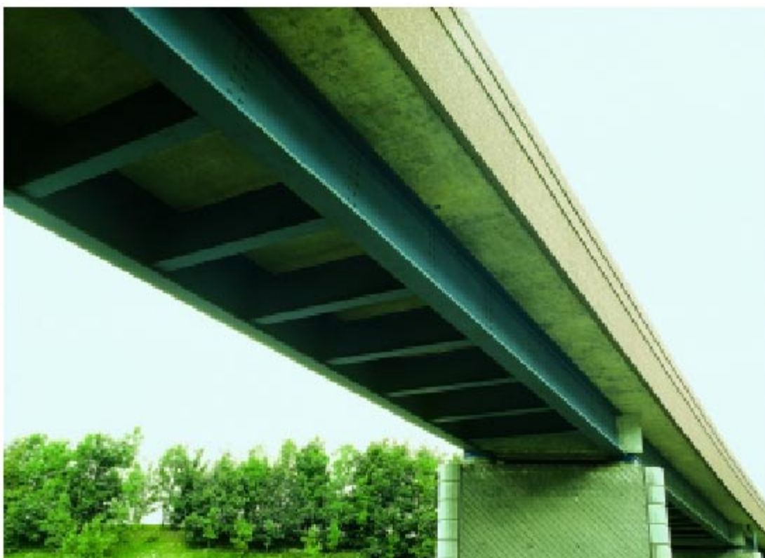
Figure 4-40: Railway bridge over the A23 motorway in Fretin, France. Four-span bridge with spans of 16,9 - 21,9 - 23,0 - 17,8. The two continuous main girders and the bracings within spans are rolled beams; the cross beams at supports are made of reinforced concrete.
