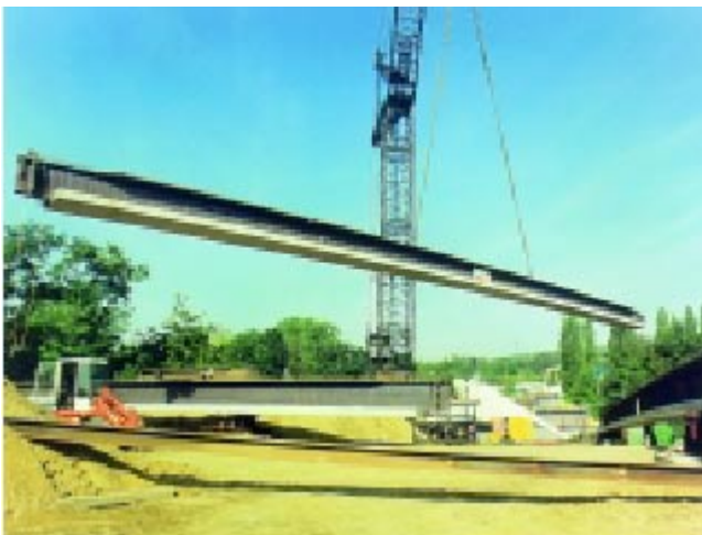
Figure 4-53: Single span bridge in Kerpen Horrem, Germany. - 41,25 m long HE 1000 A beams used for prestressed composite girders of "Preflex" type.
