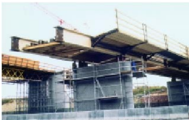
Figure 4-46: Railway bridge over the A23 motorway in Fretin, France. –Launching of the steel structure and assembled formwork.
