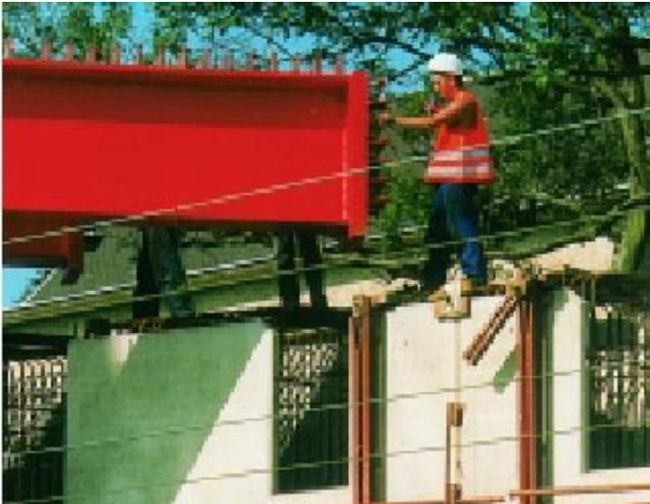
Figure 4-44: Concrete connection of main girders. - A pair of girders are lifted by crane into the recesses of the prefabricated formwork.
