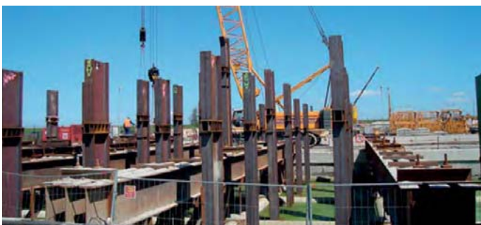
Figure 8.2: Use of HE 800 B with lengths ranging from 33,80 to 38,80m for foundations (Wilhelmshaven power plant).
