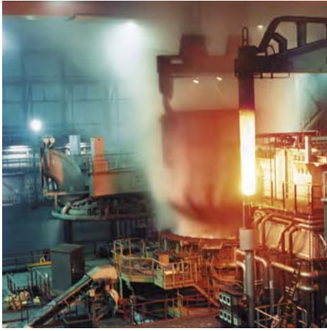
Electric arc furnace
