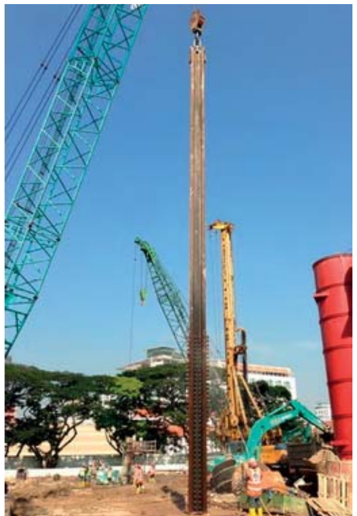
Figure 8.3: 26-metre long foundations for the top down construction method with no splicing required.
