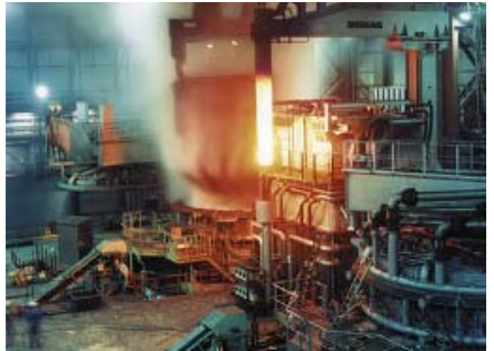
Electric arc furnace, Luxembourg
