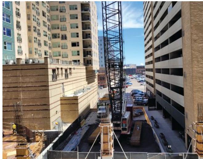
below: The construction team took advantage of an empty street adjacent to the project for crane staging and material delivery and laydown.
